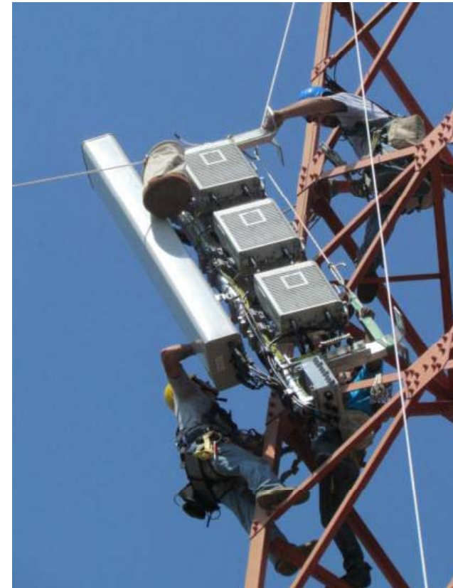
Example of an installation of a Remote Radio Configuration with the remote radio units (RRU) close to the antenna.
